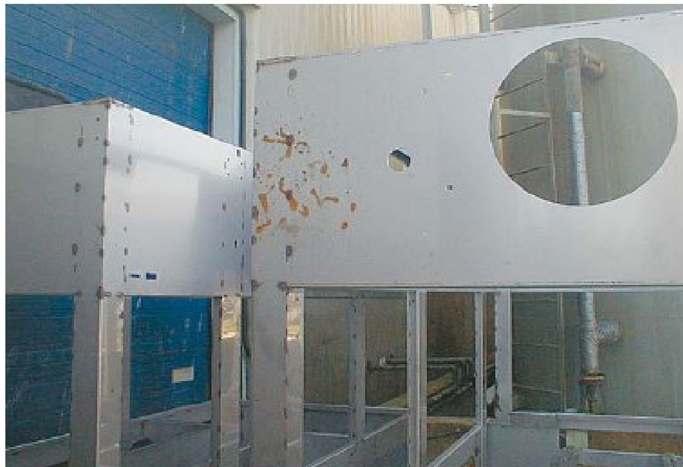
Contamination of stainless steel by iron: the example displayed is a typical case of iron contamination caused by the mixed use of iron (or steel) and stainless in the same shop without proper materials segregation. In the process of decontamination, it is important that the traces of iron are really removed and not just spread.
